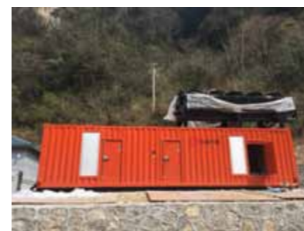
Genset in Mining Area
