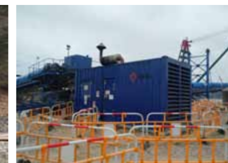
Genset Built in HK Airport
